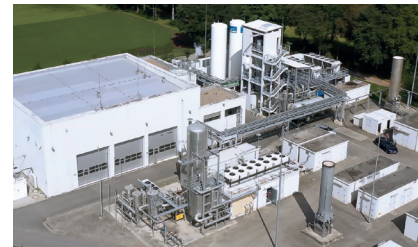
Power-to-gas plant operated by kiwi AG in Werlte, Germany
