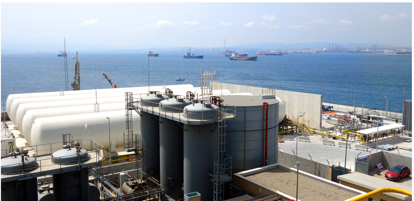
Figure 3: Small-scale LNG-fired power plant in Gibraltar
