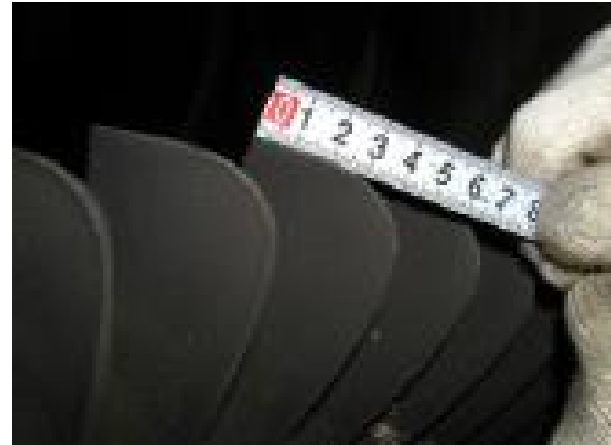
Worn turbine blade tips
