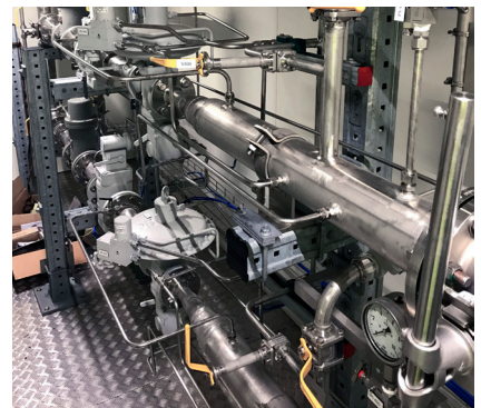
MAN PCU150 installed
