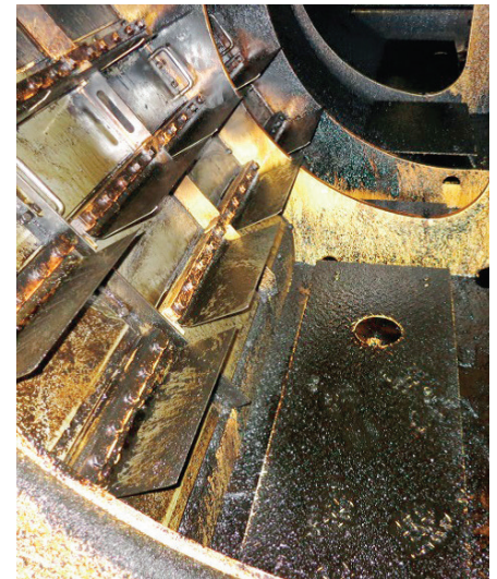
Fig. 44: Sludge and dirt accumulation in the scavenge air receiver when operating on HFO with EcoEGR
