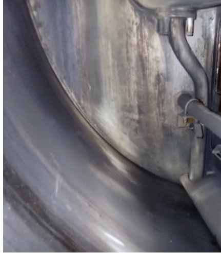
Fig. 45: ME-GI with EcoEGR. EGR unit (below EGR-cooler) with no accumulation of dirt or sludge
