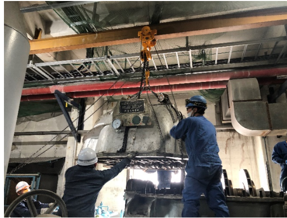
Inspection of a vacuum system by MAN Energy Solutions and JSW employees
