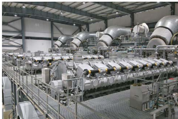
The Cambodian power plant consists of eleven MAN 18V51/60DF engines (picture source: Electricité du Cambodge)
