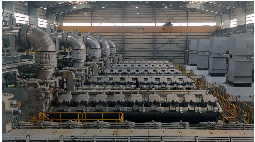
The power plant in Thakurgaon (pictured) is powered by 6 × MAN 18V48/60TS engines with a total output of around 125 MW
