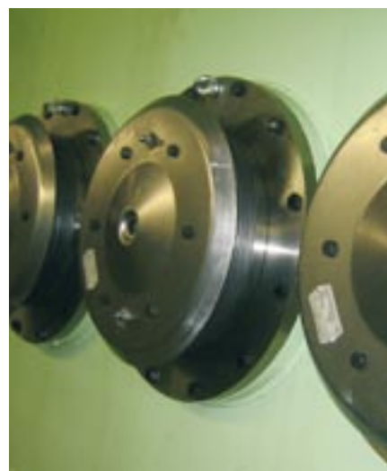
Crankcase explosion relief valves fitted on engine.
