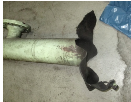
Ruptured starting air manifold
