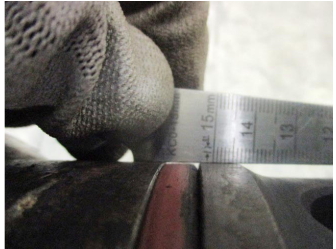
Fig. 6: Example of an O-ring with no sealing effect in the starting air valve. Please note the light between O-ring and steel ruler, which indicates that there is no sealing effect.
