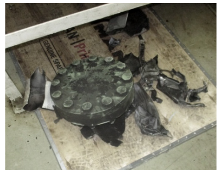
Blind flange at fore-end of the starting air manifold
