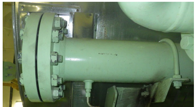
Fig. 3: Drain/venting pipe at starting air manifold at blind end (lowest point of starting air manifold).
