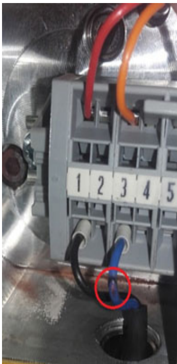
Worn-off wire insulation
